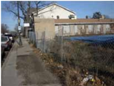
Dilapidated pedestrian facilities along Bloomington between Lake and 29th Street.
